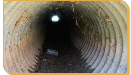
Inspect underground pipes. Conduct repairs (if necessary) and remove sediment and trash that may have collected inside.
