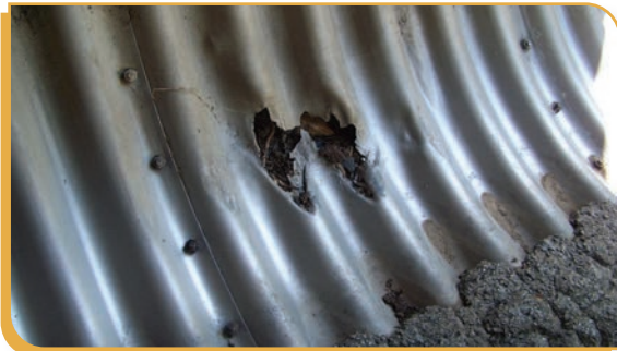
Cracked or broken pipes can cause sinkholes on your property; repair or replace damaged stormwater pipes.
