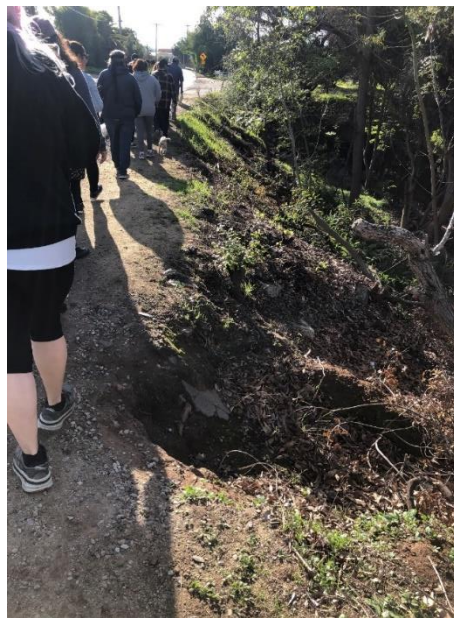
Slope and erosion west side of Foothill Drive
