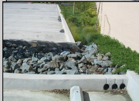
Drainage structure in top photo is obtrusive and not well-integrated into the development. In contrast, the bottom photo depicts a drainage solution integrated into project landscaping, creating an interesting mix of materials and textures.
