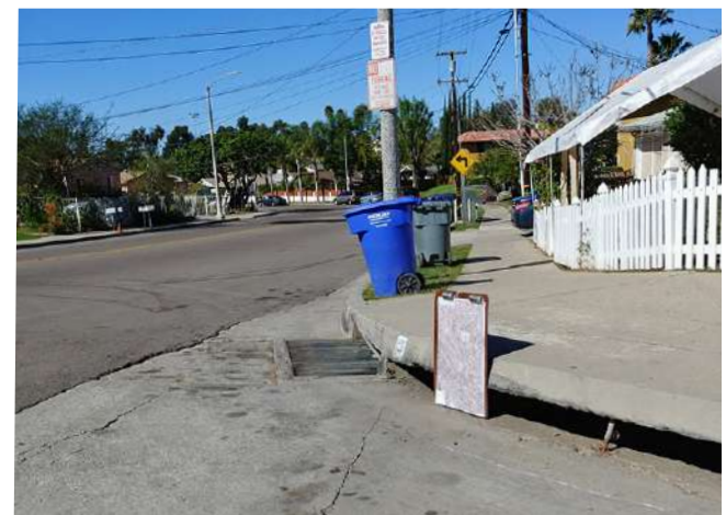
Missing curb ramps and truncated domes
